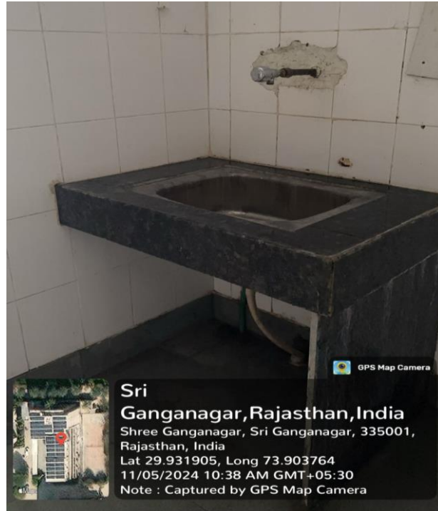
DRINKING WATER SUPPLY- BOYS HOSTEL
