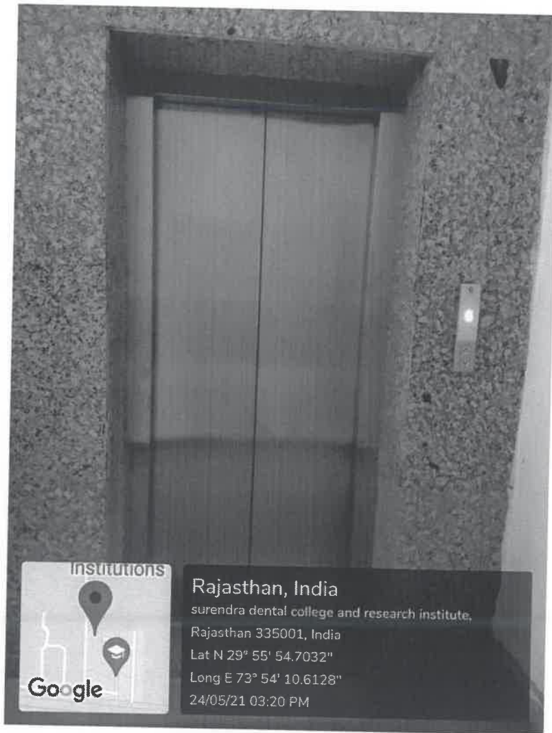
LIFT FACILITY IN GIRLS HOSTEL
